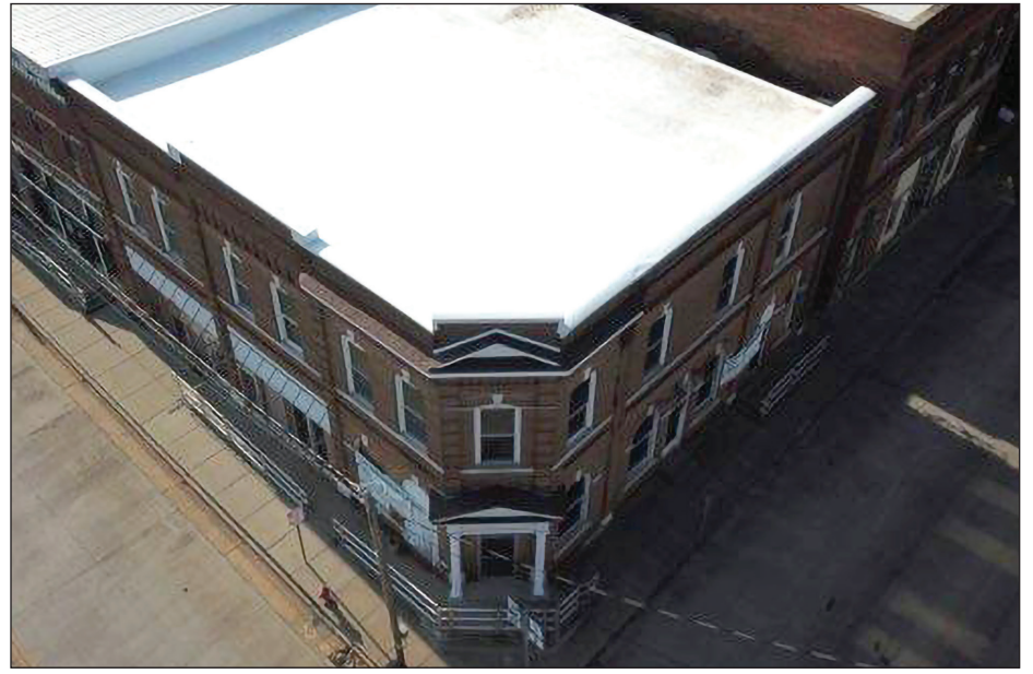
An aerial photo of the new roof recently put on the Thrive Center.
